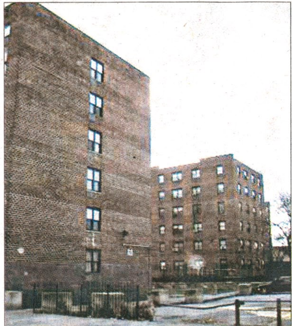
The dilapidated and crime-plagued Remeeder houses will soon get a comprehensive overhaul. (Andrew Lisa)
